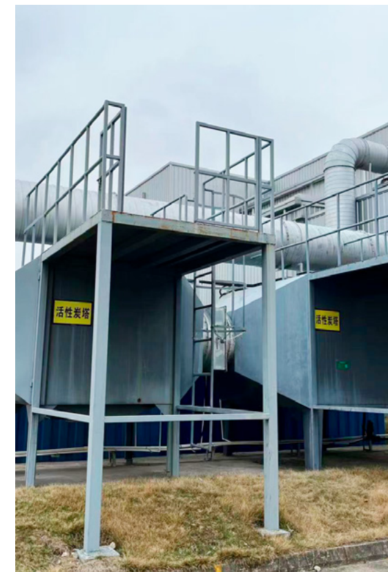
Double activated carbon facility at GC Suzhou
